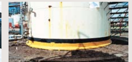
Anti-corrosion around the base of tanks.
