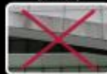
Streaking (Silicone Sealant)
