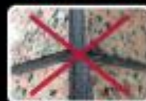
Poor UV resistance – Sealant cracking (PU Sealant)
